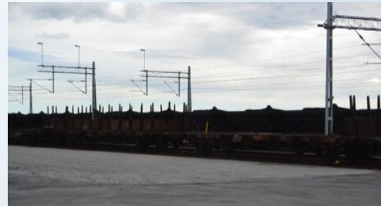
PUBLIC ACCESS ELECTRIC RAIL
